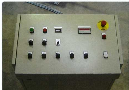
BA-D control panel.
