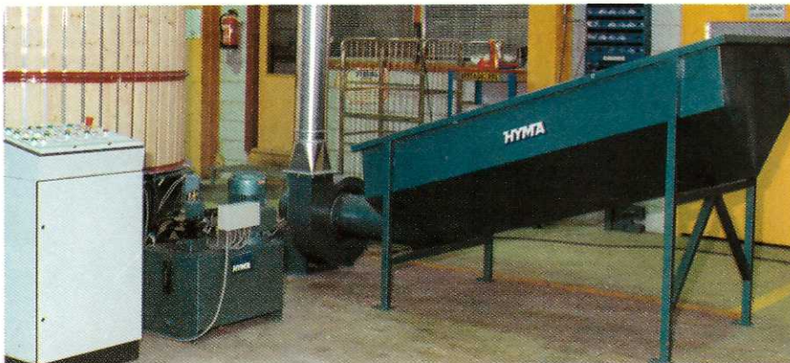
Filling the silo from sack emptying station.
